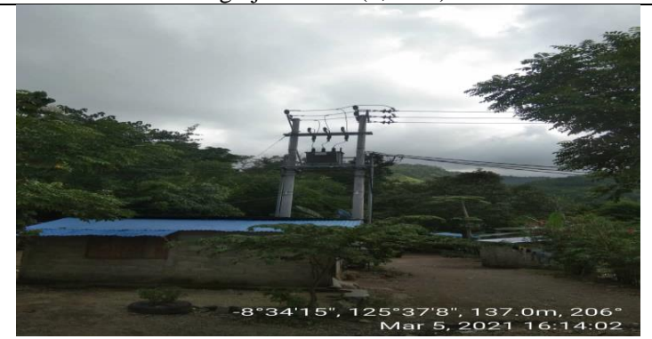
Electric Pole (350 m)
