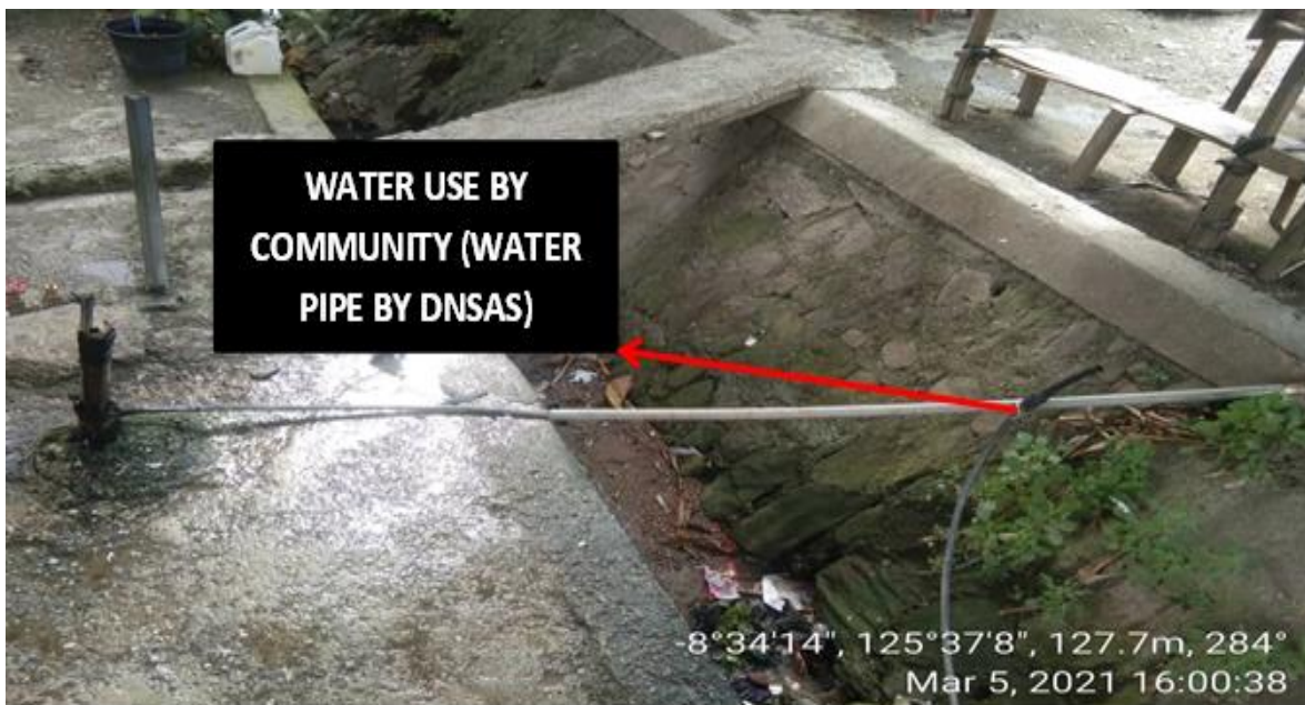
Figure 22. Water Pipe (DNSAS Clean Water)
